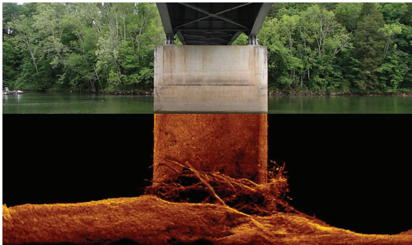
Figure 11. Drift at pier foundation easily detected using sector scanner sonar.
